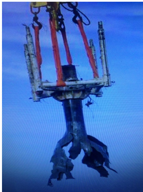
Fig. 5 Lifting of oil pipes from the seabed during a decommissioning of an oil field between Scotland and Norway, 2006. Image courtesy of John Kettles, Blast Design.
